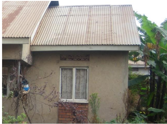
Figure 2. Permanent ventilators on windows and doors
