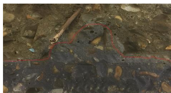
M 0.4-crack width 0.1 mm
