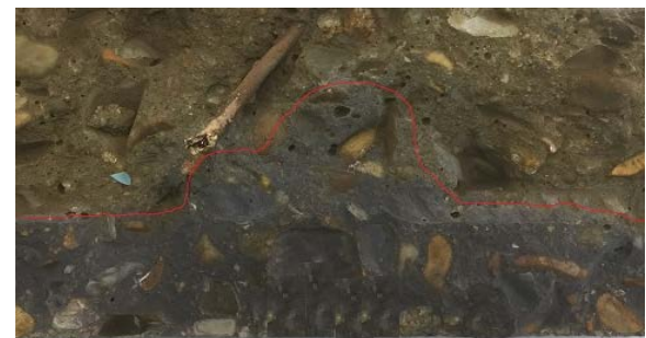
M 0.4-crack width 0.1 mm
