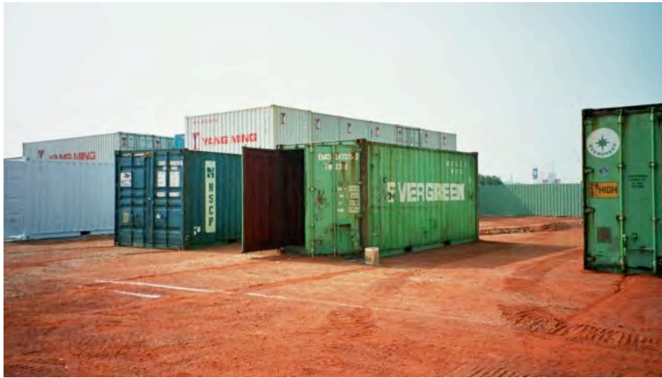
Case study 1. The Flight (2003). Construction site with the container allocated for the installation
