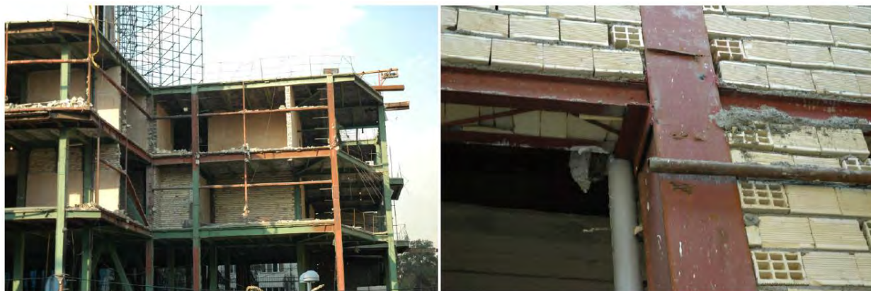
Figure 2: Low building quality in Iran.
