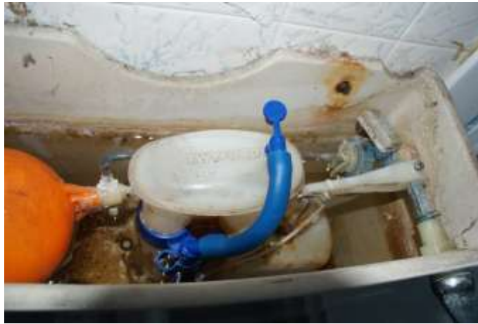
Figure 3: Ecobeta® cistern retrofit
