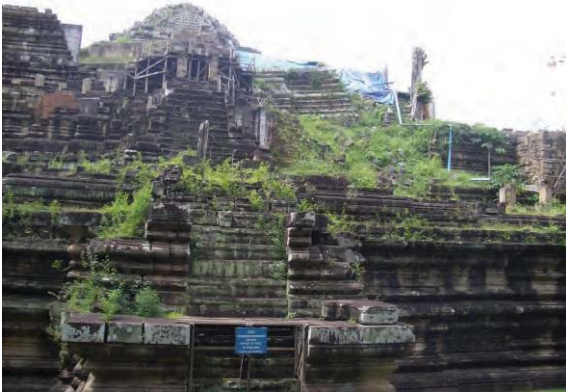
Figure 4(a): Part of a temple at Ankor Wat under reconstruction in a project which started in 1908
