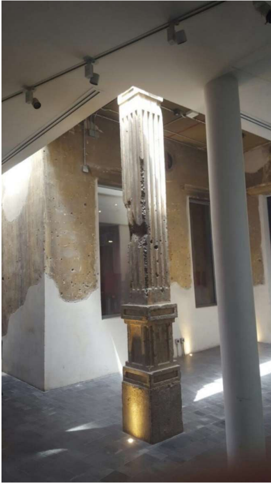
FIG. 18 Polished walls, new lighting, refurbished floor, an older and a more recent pillar (source: HMA)
